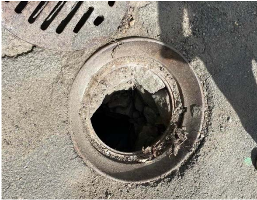
Figure 4 - In-line catch basin at 5 School Street.
