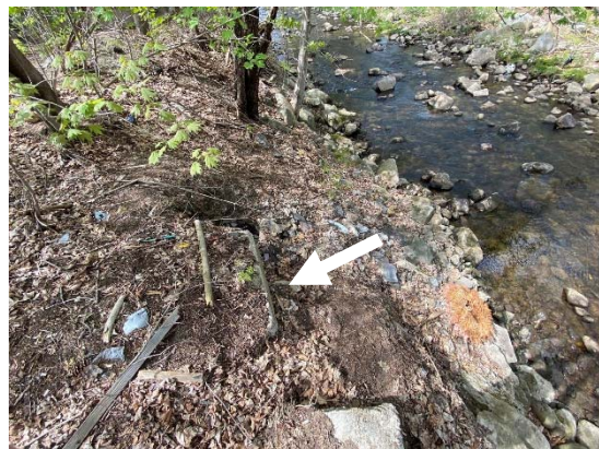
Figure 5 - Existing NHDOT outfall from Main Street.
