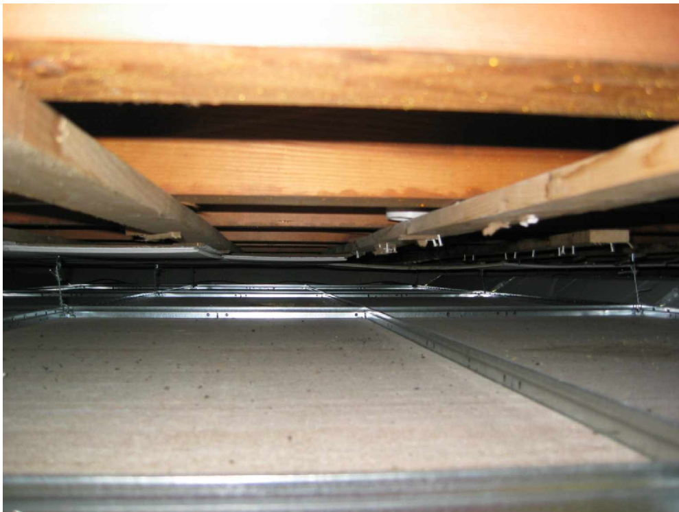
PHOTO 11 - TYPICAL VIEW OF 2-1/2 x 13 RAFTERS LOOKING FROM THE OBSERVATION OPENING PERPENDICULAR TO SPAN (Room 211)
