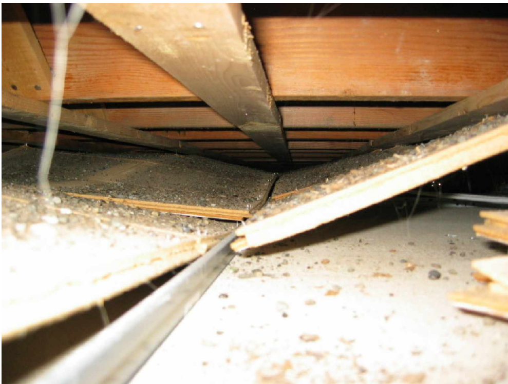
PHOTO 7 - TYPICAL VIEW OF 1-1/2 x 13 RAFTERS LOOKING FROM THE OBSERVATION OPENING PERPENDICULAR TO SPAN
