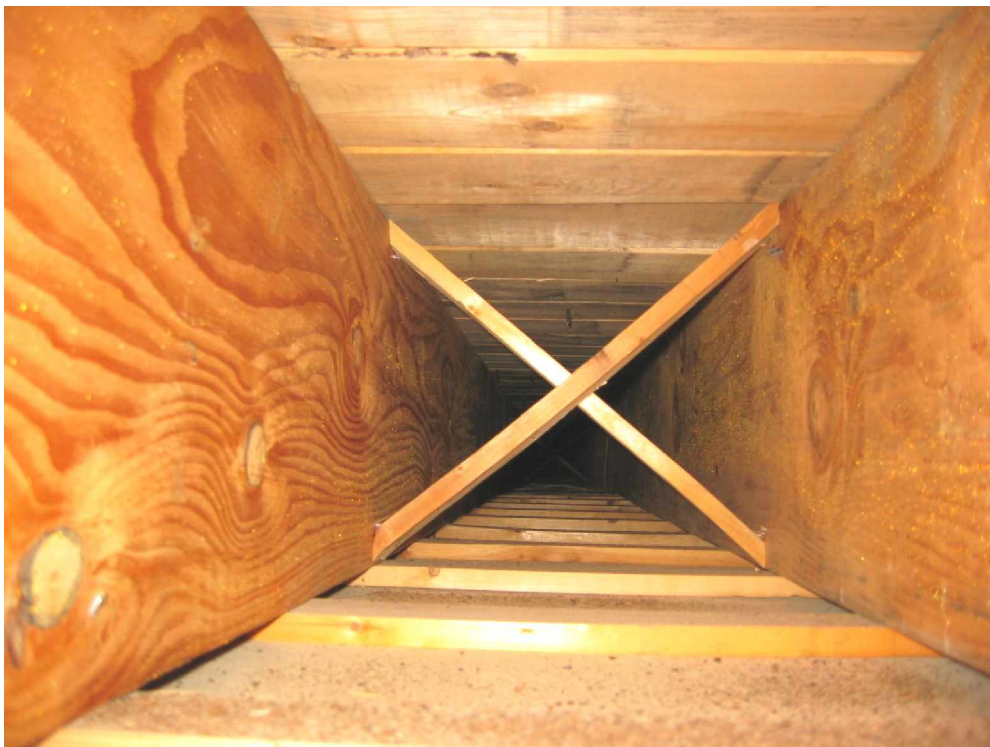
PHOTO 5 - TYPICAL VIEW OF 1-1/2 x 13 RAFTERS LOOKING FROM OBSERVATION OPENING IN OPPOSITE DIRECTION FROM ABOVE (Room 207)
