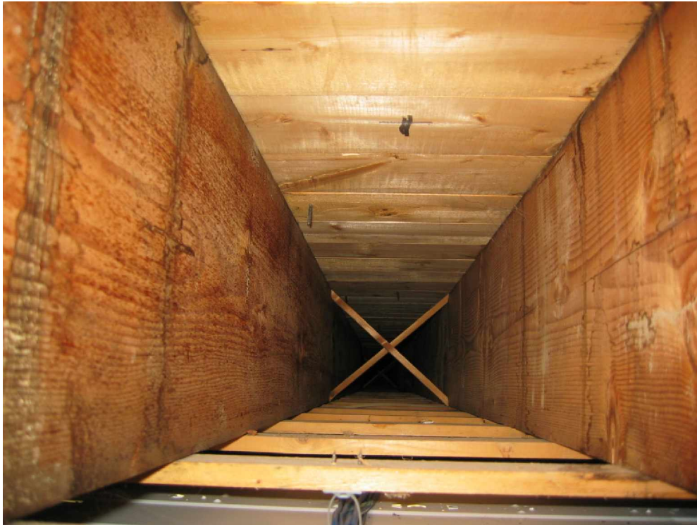
PHOTO 10 - TYPICAL VIEW OF 2-1/2 x 13 RAFTERS LOOKING FROM OBSERVATION OPENING DOWN THE BAY - OPPOSITE DIRECTION FROM ABOVE (Room 211)
