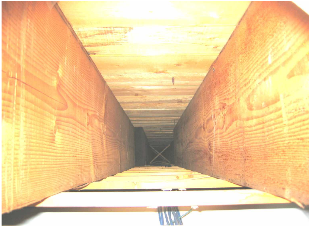
PHOTO 9 - TYPICAL VIEW OF 2-1/2 x 13 RAFTERS LOOKING FROM OBSERVATION OPENING DOWN THE BAY (Room 211) NOTE OVERLAPPING BEARING CONDITION OF 2-1/2x13 RAFTERS
