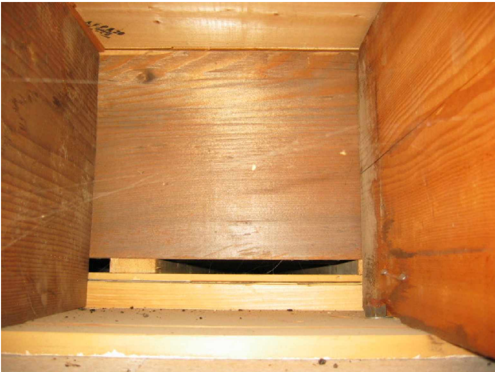
PHOTO 13 - TRANSITION FROM ROOM 217 TO ROOM 218 DIRECTION OF SPAN CHANGES
