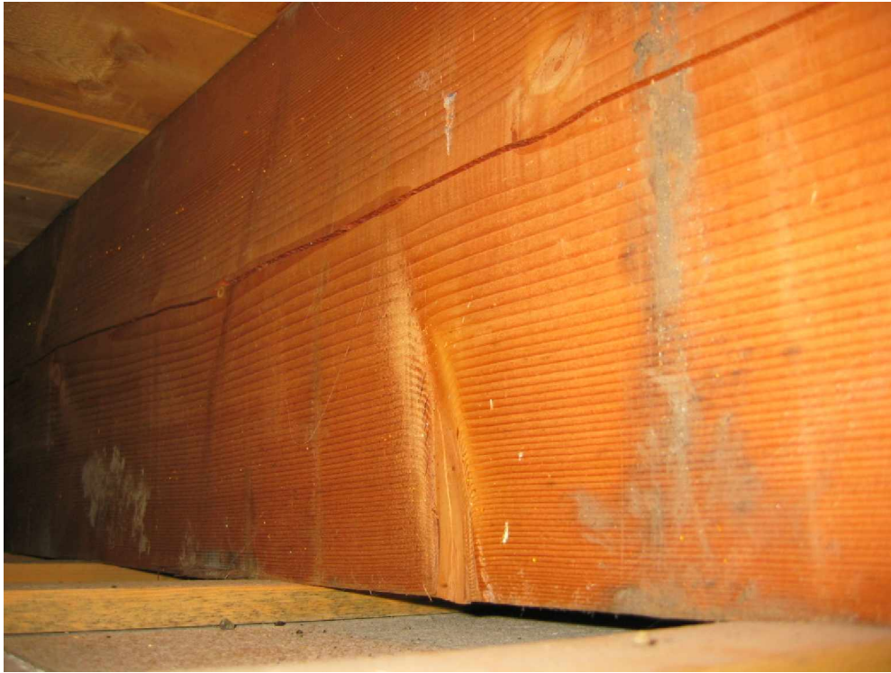
PHOTO 12 - TYPICAL (WHERE FOUND) CHECK IN 2-1/2" x 13" RAFTER
