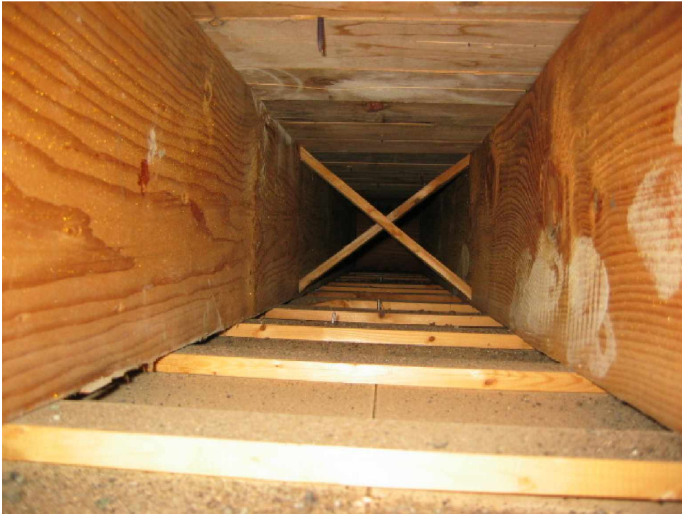
PHOTO 6 - TYPICAL VIEW OF 1-1/2 x 13 RAFTERS LOOKING DOWN THE BAY FROM OBSERVATION OPENING
